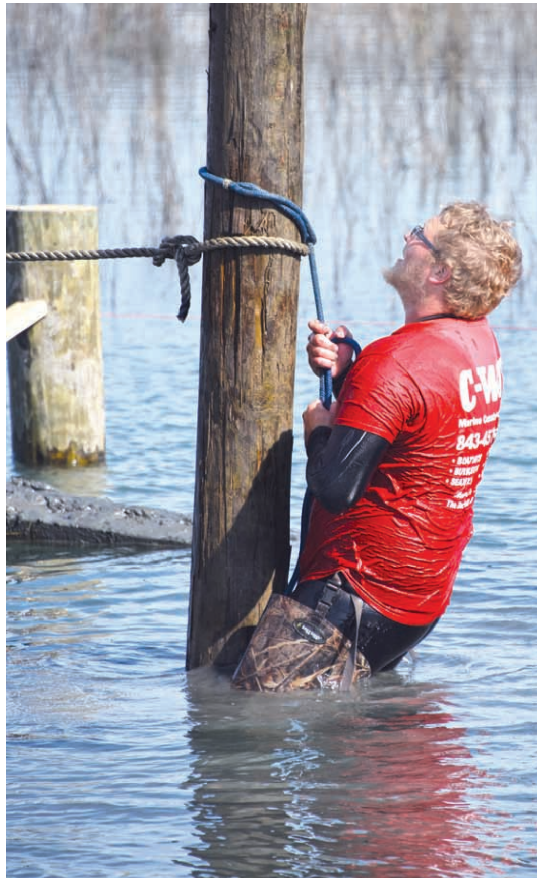
Rob Lupine of C-Way Marine sets a piling for the Pawleys Island Chapel Tanya Ackerman/Coastal Observer
